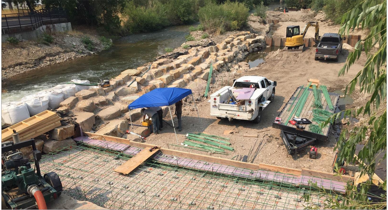
Weber River diverted to the west as construction continued on the eastside Kayak Park.
