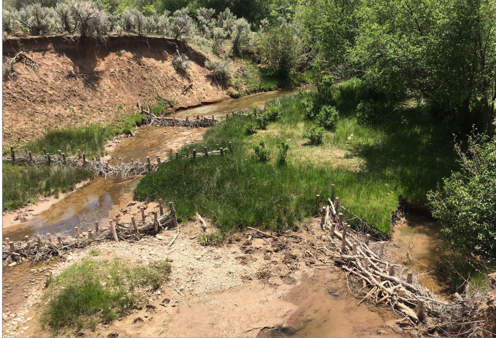
BDAs retain sediment in Fish Creek, providing new areas for vegetation to emerge. June 2021
