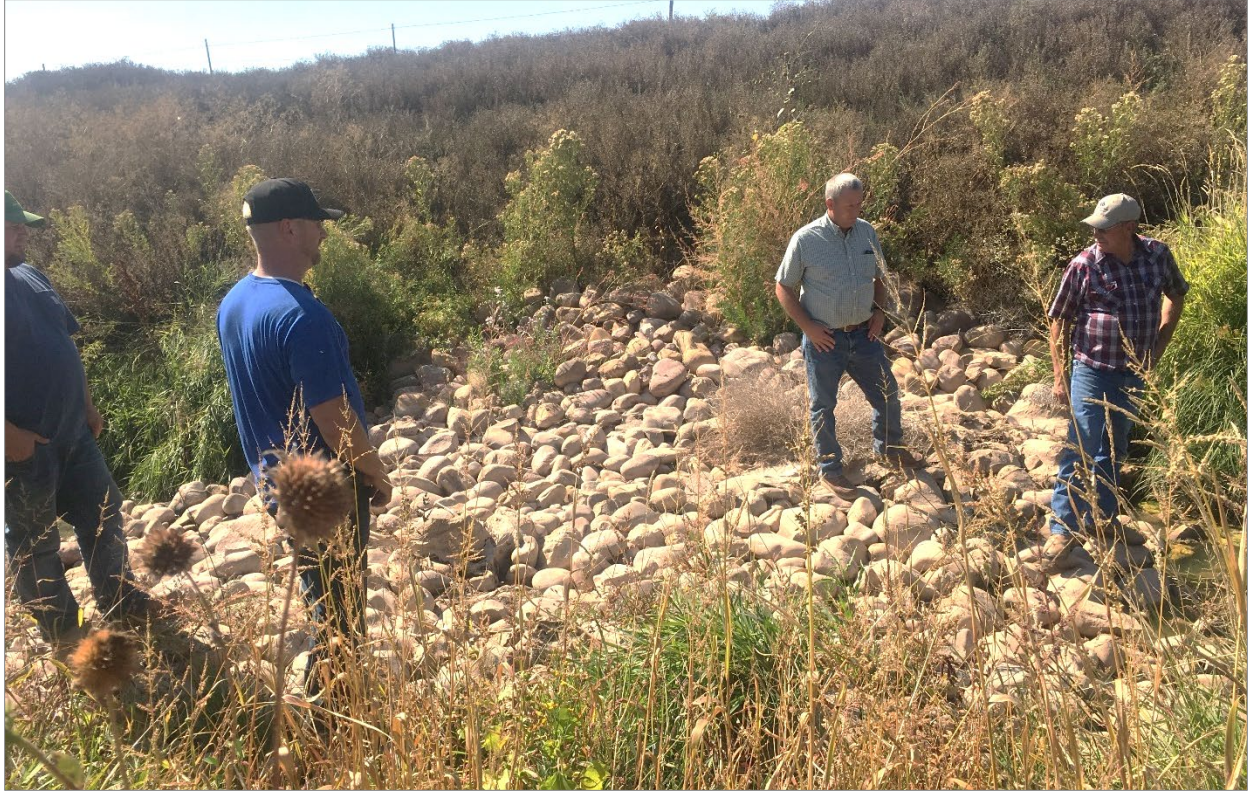
Uintah Conservation District, NRCS, UDWR, and landowners discuss options to address downcutting and erosion in the Bullock Canal that feeds into Pelican Lake.
