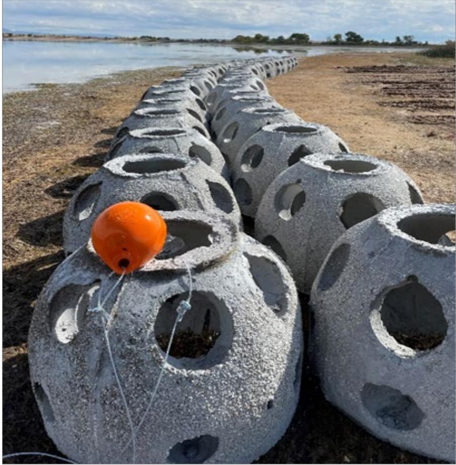
Reef ball structures to create a living shoreline and reduce both turbidity and wave action on this southern shoreline.
